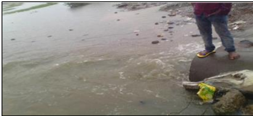
Sea Water intrusion point
