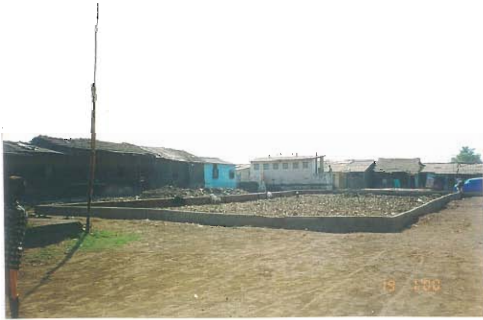
Plate 7: Extension of the Project capacity after completion of the site development by MCGM
