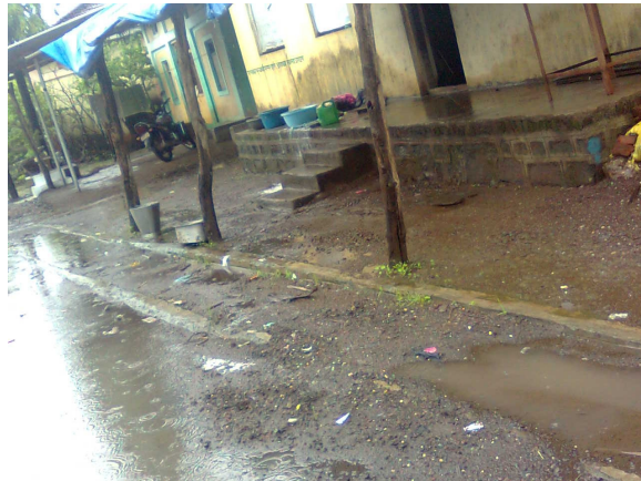
Fig No. 6.6 Siltation in existing storm water drains in RTDZ at Akloli.
