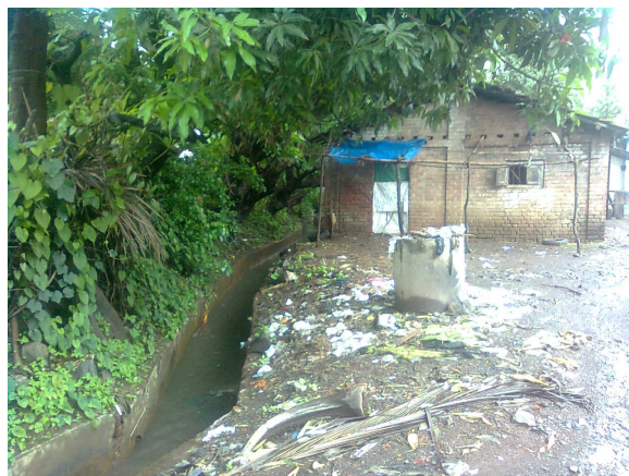
Fig No. 6.7 Garbage mixing into existing storm water drains at Vajreshwari.
